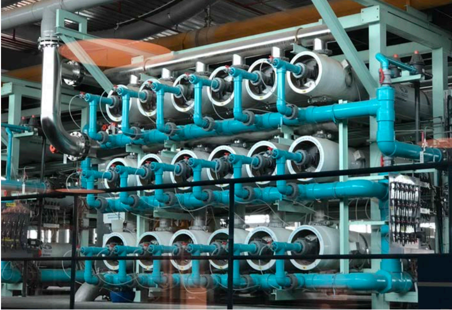
NEWater treatment facility.
