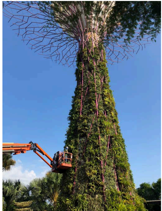
Giant cranes hoist workers up to add more plants to one of the Super Trees.
